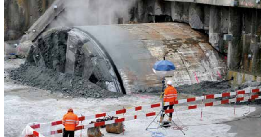
Tunnelling machine at work: Break-through of the drilling head with its rotating bits.
